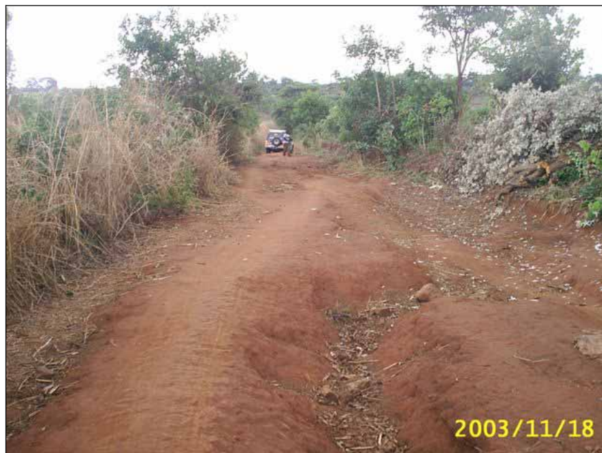
Figure 4.3: Chinjala Road, Zambia – Last maintained 10 years ago (RuralNet, 2004)
