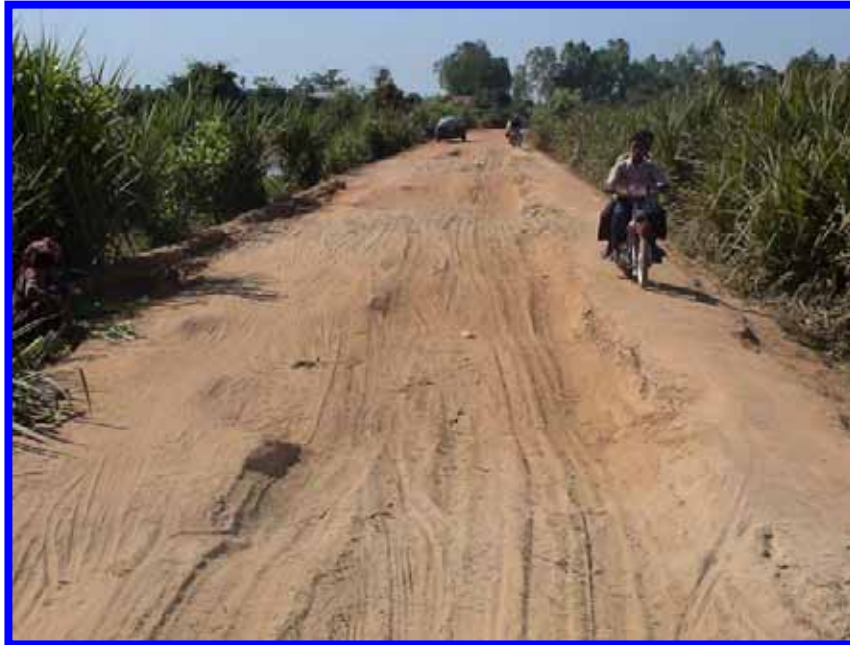
Figure 1 – A donor funded project gravel road within 2 years of maintenance cessation (photographed in the dry season! – impassable to motor cars)
