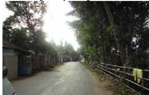
Fig.10 - Road furniture, trees, telegraph posts etc. on RHS are gradually leaning towards the river.
