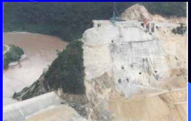
The Yunnan Manwan waterpower station is at middle reach of Lancanjiang river.
