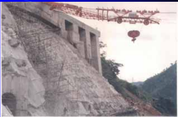
After anchor cable support was completed, the gigantic cable crane is restarted to run.
